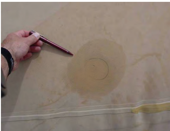
Figure 3. Example of a Class I leak
