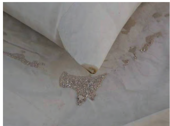
Figure 7. Example of a Class I corner leak
