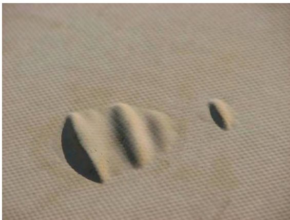
Figure 10. Example of blister in panel
